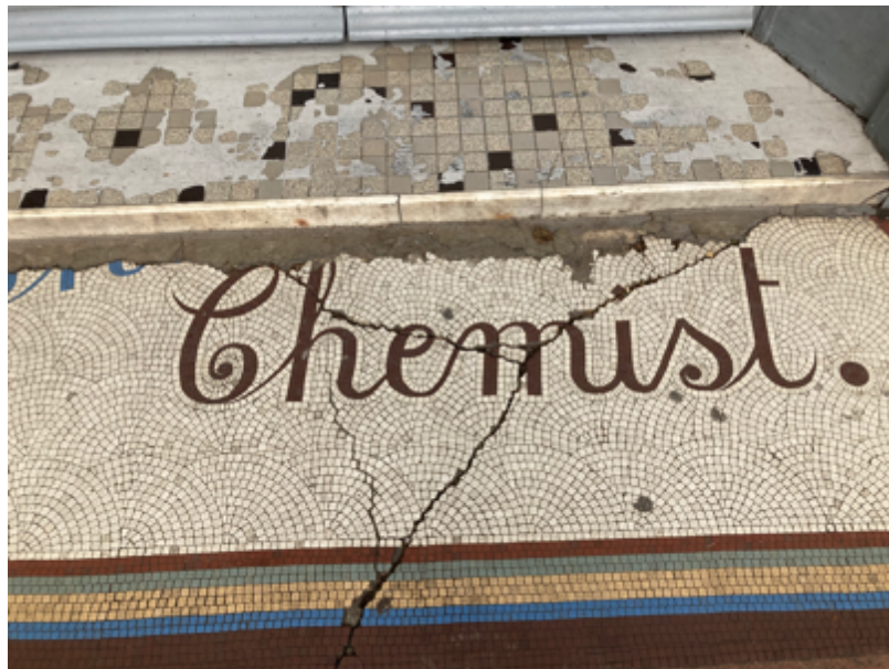
Figure 24: Damaged mosaic threshold at Broadway Mansions
