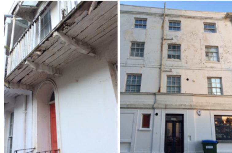
Figure 75: Examples of poorly maintained buildings on Warwick Road
